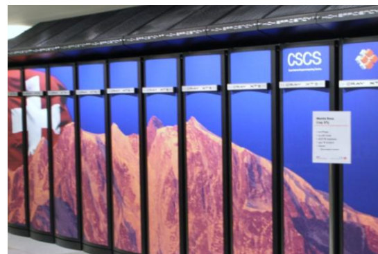
Abbildung 5: Serverracks am CSCS in Manno
